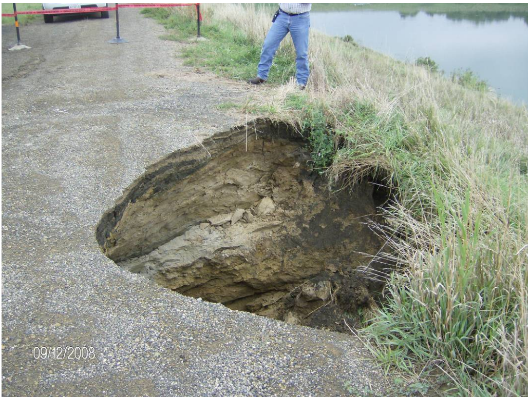
View of Sinkhole Looking Southeast Along Dike
