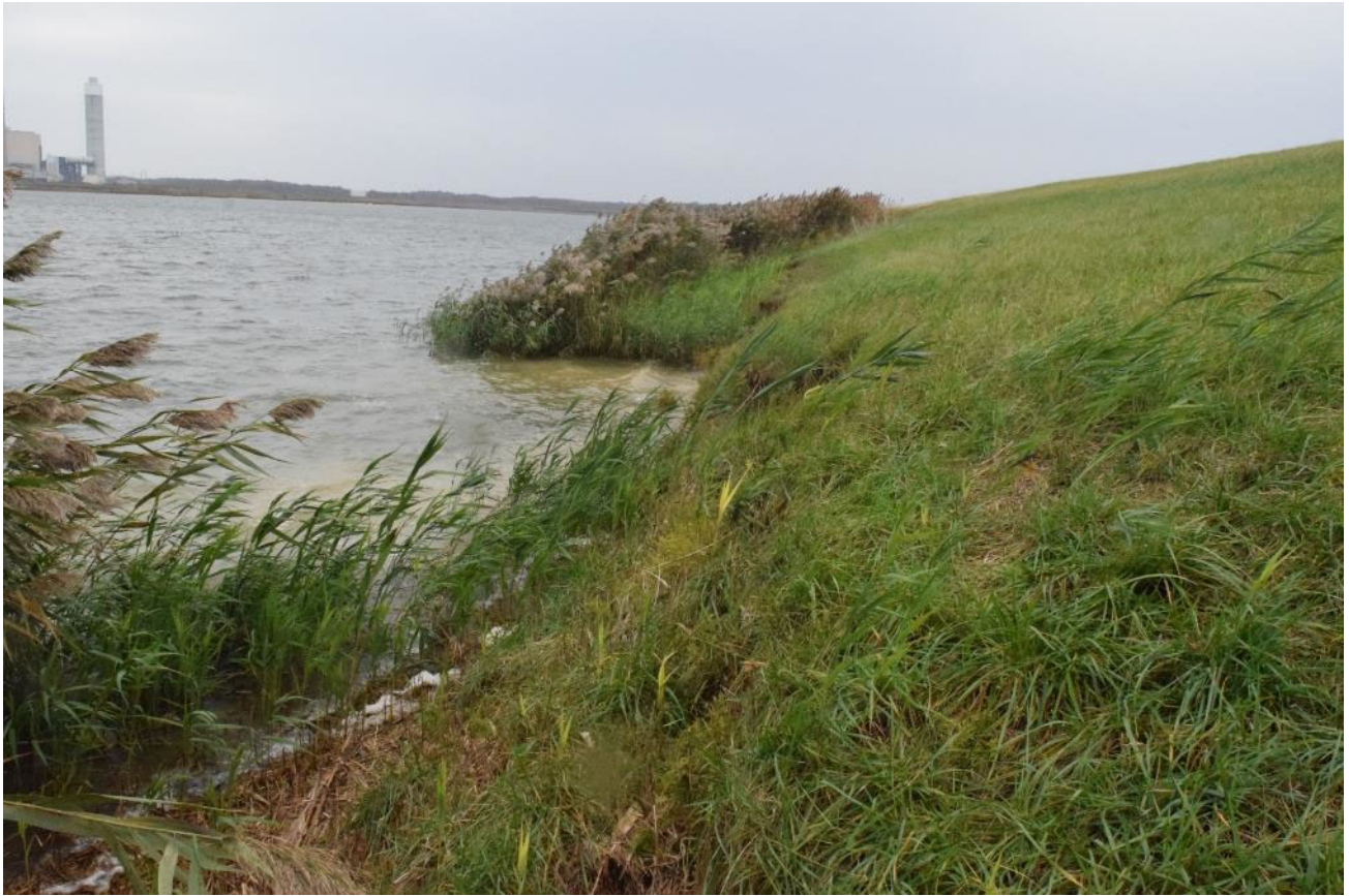
Sloughing & bench erosion of upstream slope –primary pond – repair
