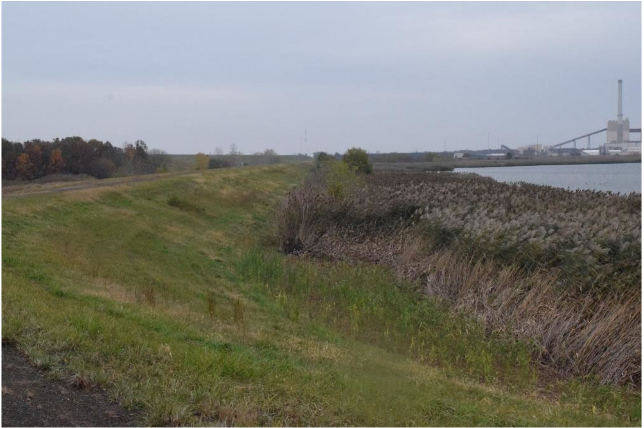
West upstream slope – remove woody vegetation
