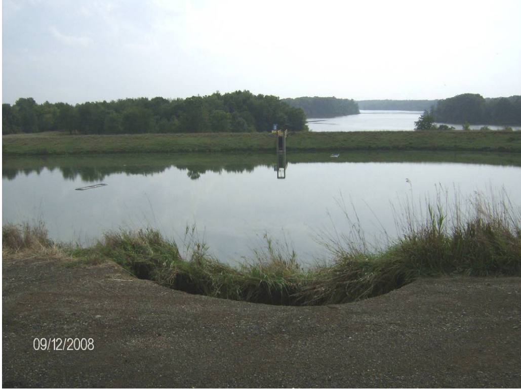
View of Sinkhole Looking Southwest Towards the Secondary Pond and Lake
