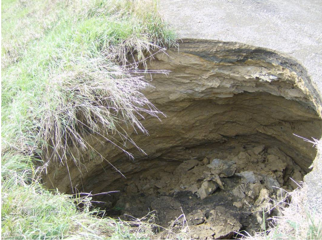
Close-Up of Sinkhole
